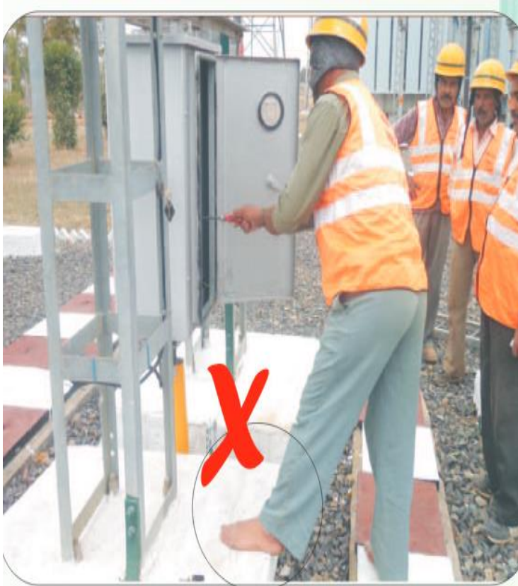
Without shoes in switching yard
