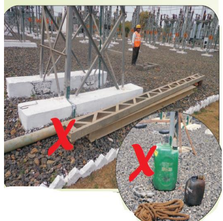
Do not leave unwanted materials in switching yard
